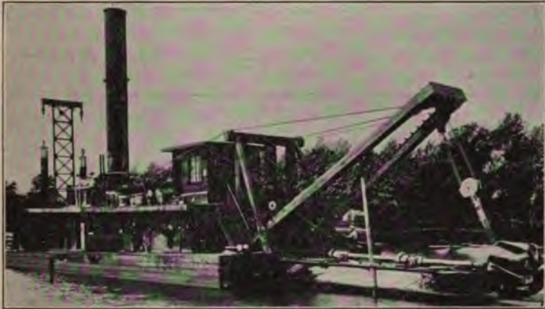
View of Hydraulic Dredge showing Cutter, Cutter Frame and Gantry and Spuds and Spud Gantry.
